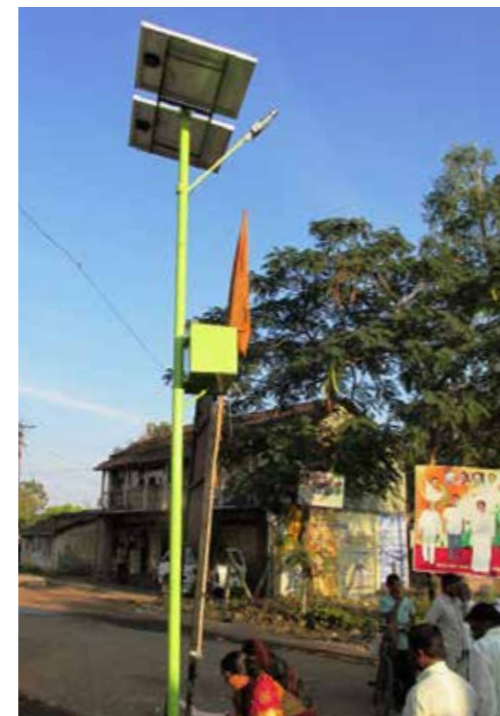
Nine Solar Street Lights installed in different locations at Kanagala on 16 November, 2013
